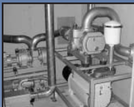
Compact Oil Mist Exhaust Filter Mounted on a Vacuum Pump
